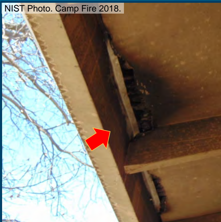
Failure: eave at fascia board
