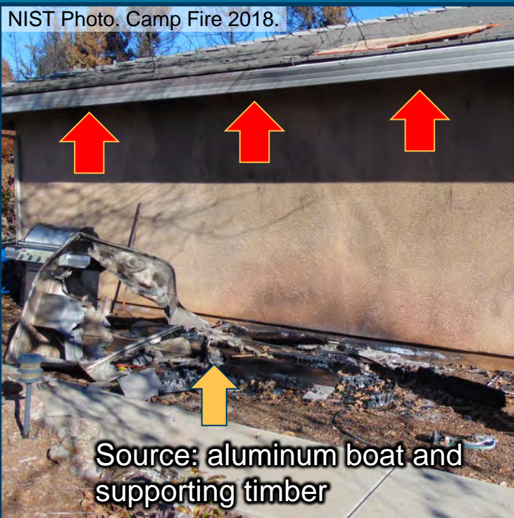
Failure: multiple locations along eaves
